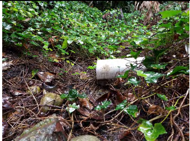
Stormwater from 1818 70th Avenue SE.
